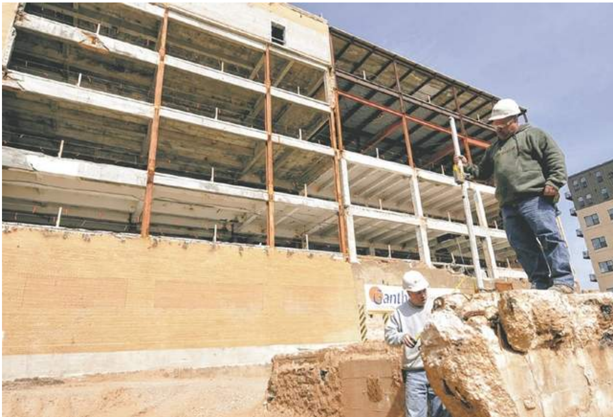
The WaterMark project in downtown Green Bay is seeing some activity as workers with Ganther Construction|Architecture begin site survey work. Site Supervisor Joe Hurzeler, left, works with carpenter Steve Dietzen last week. / Jim Matthews/Press-Gazette
