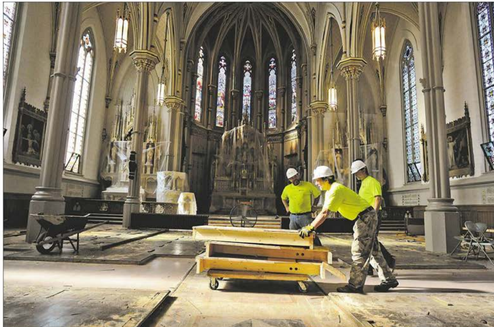
Don Moore of Ganther Construction pushes a dolly July 20 loaded with material that was moved from a riser in the sanctuary at Most Blessed Sacrament's St. Mary's site. Rick Standrik and Al Hollis Jr. walk out with him to dispose of the materials. During renovations crews have found coins, a prayer book and a rosary lost in 1961. JOE SIENKIEWICZ/OF THE NORTHWESTERN
